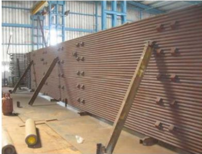
PROJECT : LALITPUR (660MW)
