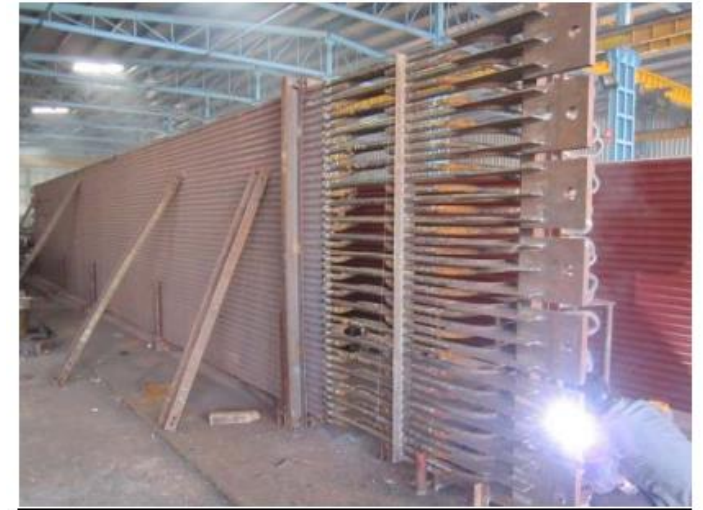
PROJECT : YERAMARUS (800 MW)
