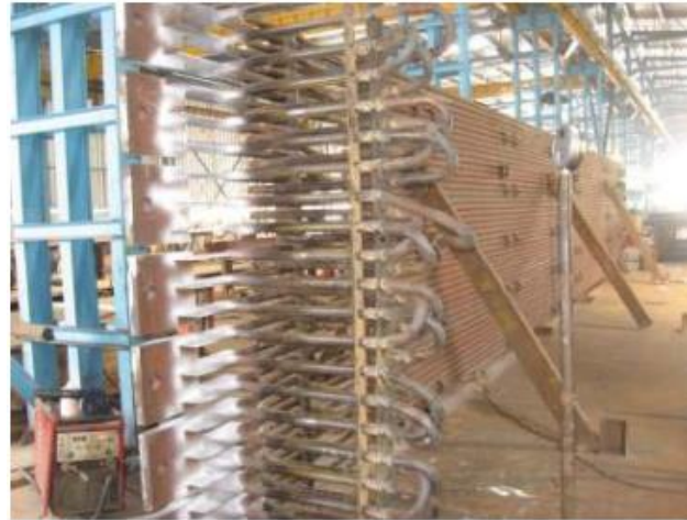
PROJECT : LALITPUR (660MW)
